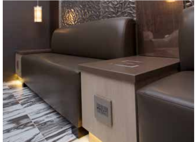
adorne standard Furniture Power Center installed in a lobby.
