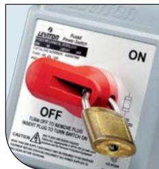
Handle with padlock installed
