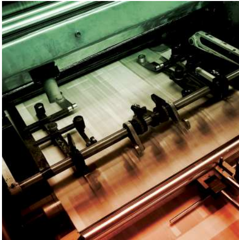
Lexium SD3 drive controlling a printing machine
