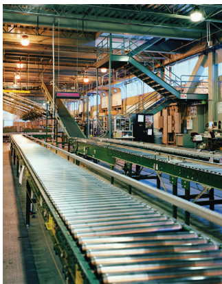
Material handling application
