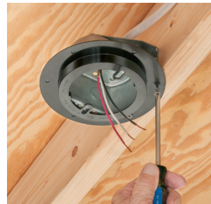
...through the device holes or flashed-over holes to hold it in place during drywall installation.
