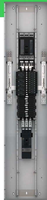
800A NF MB Panelboard with 600A SFB
