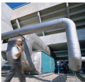
Air handling unit
