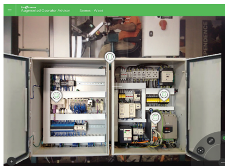
Virtually-open electrical cabinet
