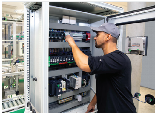
General machine control
